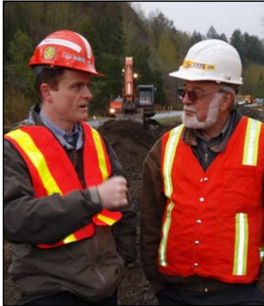
James Baxter/Photo Barry and Fred Feistmann of Emil Anderson survey the $3.1 million Wilson Road dike expansion. This important project will help protect this vulnerable neighbourhood from future flooding.
